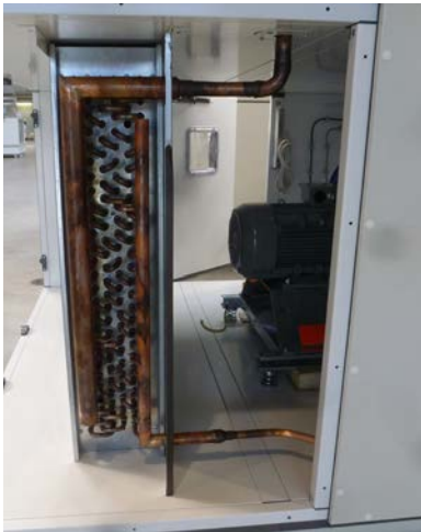
Condenser in an air handling unit
