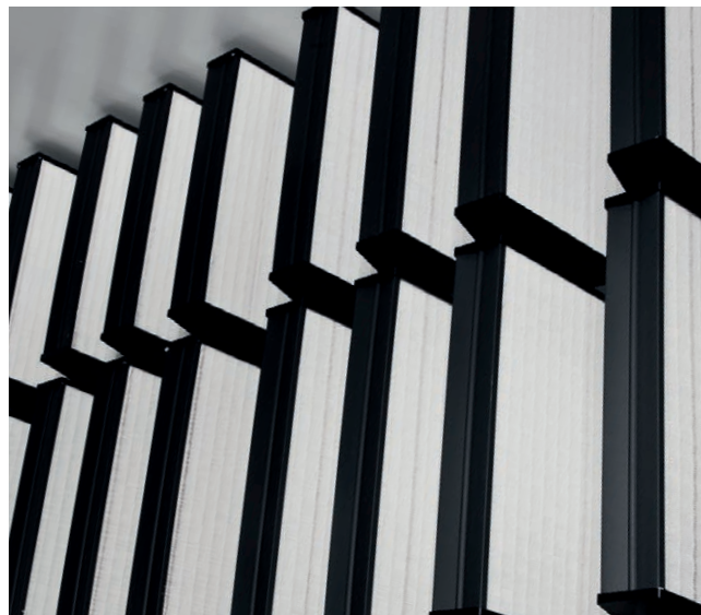
Filter inserts in an air handling unit
