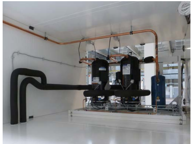
Compressor in the air handling unit
